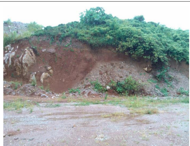
FIGURE 2 | Red clay slopes encountered during highway excavation in the study area.
