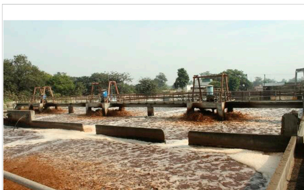
FIGURE 7 The aeration tank overflow is processed further with a secondary clarifier to remove suspended active biomass.
