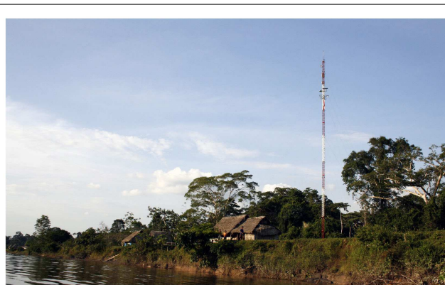
FIGURE 2 | Infrastructure of solar panels and tower installed in an isolated health posts.
