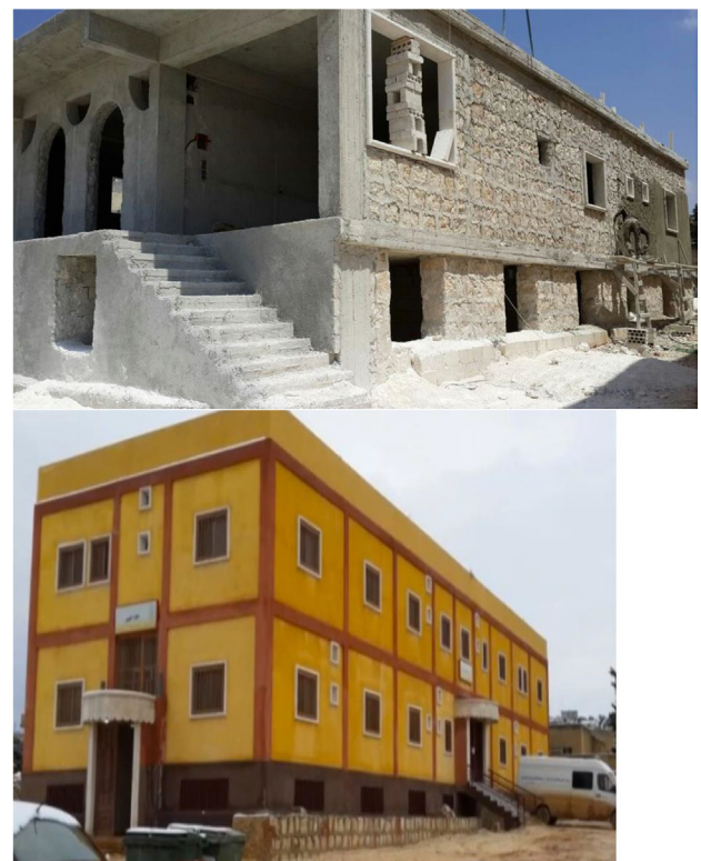
FIGURE 2 | Picture of Brotherhood Medical Center (BMC) at Initial Phase of Construction and BMC Main Hospital Building Post-Construction.
