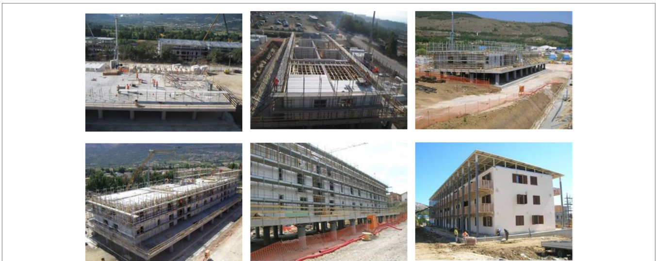
FIGURE 11 | Work phases (“Piano C.A.S.E.”) (from the top left to the bottom right) day 1: work initiation; day 4: positioning of the slab modular panels; day 7: first floor completed; day 11: second floor completed; day 17: structure completed; day 73: building ready to be occupied (courtesy of Nidyon Costruzioni).
