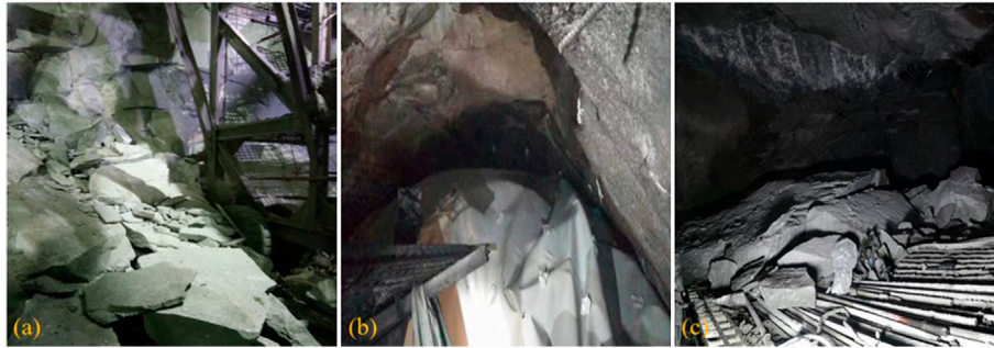
FIGURE 1 | Rockburst disasters occurred at Paoma mountain No. 1 tunnel.
