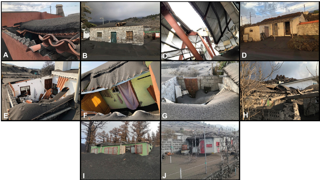
FIGURE 5 Collapsed roofs of primary structures as observed in the field. (A) tiled single pitch irregular plan/composite design roof with one storey regular masonry (MS, zone L), (B) tiled two or more pitches, regular plan and simple design, with one storey regular masonry (MS, zone B), (C) two or more pitches, metallic, regular plan and simple design, with one storey, mixed structure (WE, zone L), (D) tiled two or more pitches, regular plan and simple design, with one storey regular masonry (MS, zone H), (E) pitched roof of fiber cement/zinc, irregular plan/composite design roof with one storey regular masonry (WE, zone L), (F) single pitch of fiber cement/zinc, regular plan and simple design roof with one storey regular masonry (WE, zone L), (G) single pitch metallic regular plan and simple design roof with one storey regular masonry (WE, zone L), (H) tiled two or more pitches, regular plan and simple design, with one storey irregular masonry (MW, zone L), (I) single pitch metallic irregular plan and composite design roof with one storey regular masonry (WE, zone TTLL), (J) flat fiber cement/zinc regular plan and simple design roof with one storey regular masonry (WE, zone B).
