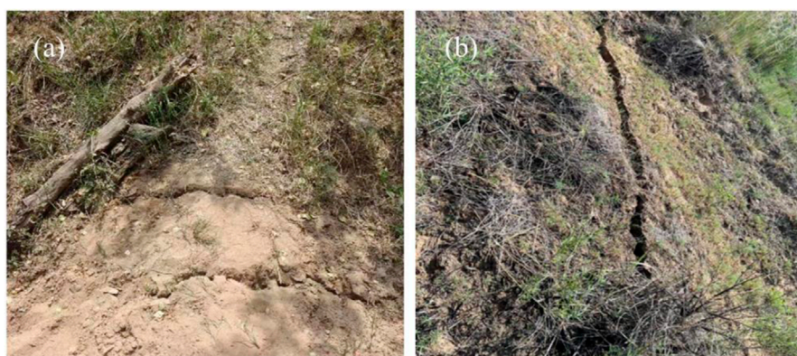
FIGURE 17 Surface fractures: (a) surface fracture 1; (b) surface fracture 2.
