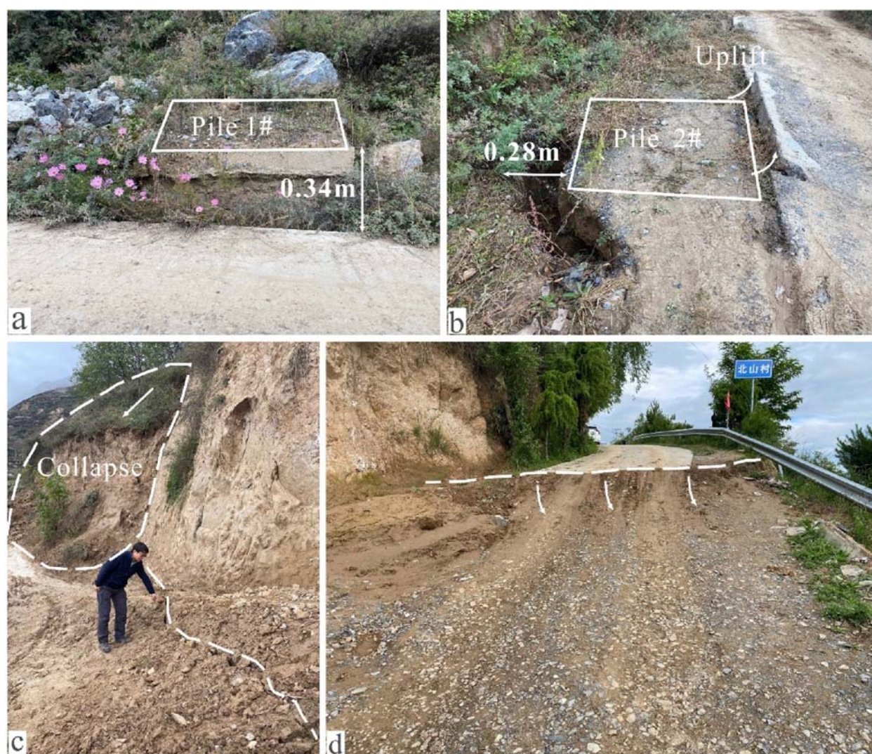
FIGURE 8 Deformation of cracks in the road area. (a,b) Deformation of piles; (c,d) Deformation of road.
