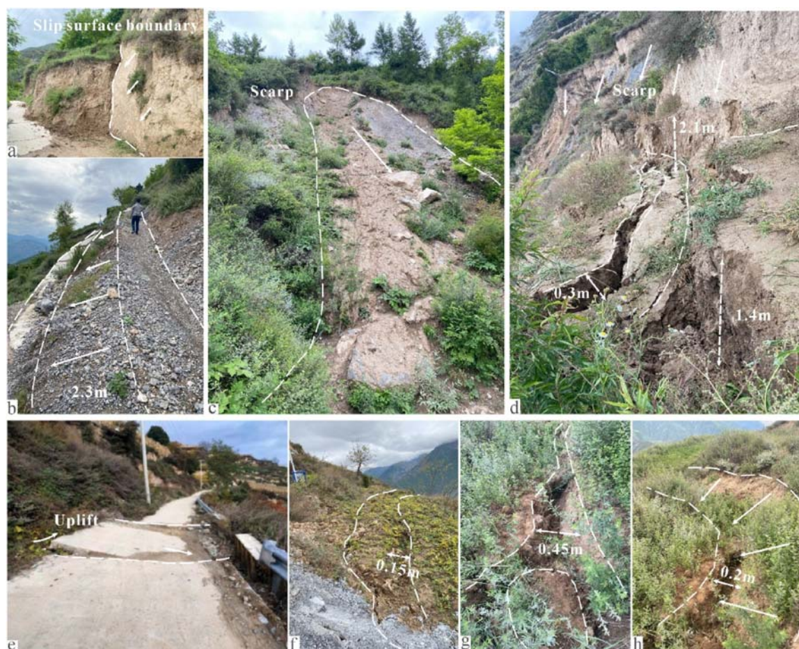
FIGURE 3 Deformation of cracks based on field investigation. (a) Slip surface boundary; (b,e) Deformation of roads in the landslide; (c) Collapse; (d,f–h) Deformation of cracks.
