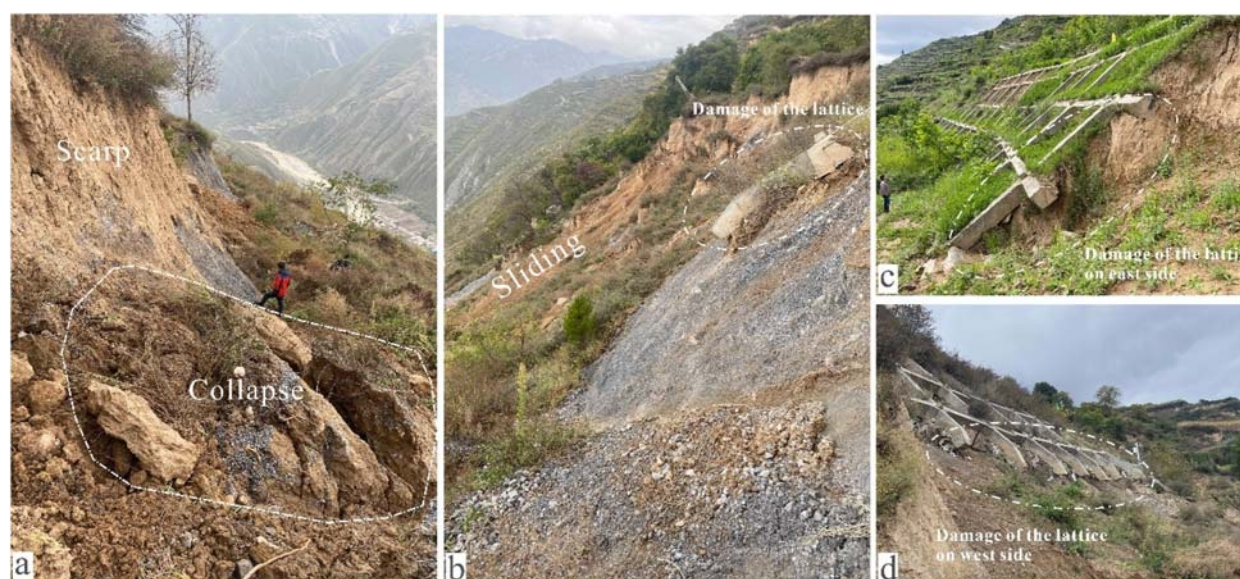
FIGURE 9 Deformation on the front edge of the landslide. (a,b) Collapses on the front edge of the landslide; (c,d) Damage of the lattices.
