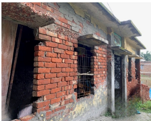
FIGURE 4 Salinity affecting the local healthcare center (Community Clinic). Source: Authors during field work.
