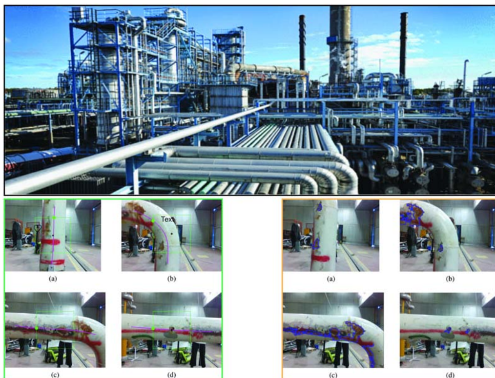
FIGURE 8 Industrial pipeline anomaly detection (reprinted with permission from Roos-Hoefgeest et al., 2023 Copyright © 2023, IEEE). (a–d, green border) Pipeline tracking: pink line marks the central axis, green guides the drone. (a–d, orange border) Corrosion detection on RGB pipeline images, defects in blue.
